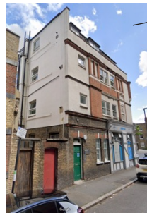
York House has a complex façade. Windows, ventilation and flat roof insulation could be priorities along with PV.
