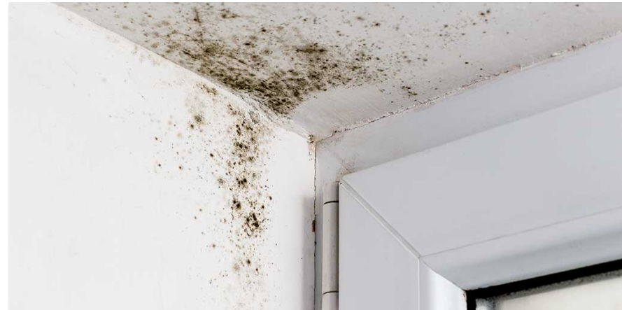
Example of mould growth in apartment ceiling due to moisture build-up and poor ventilation strategy
